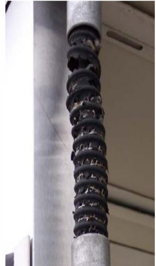
Deterioration of Stage II Connection hose, courtesy of VA DEQ Piedmont Office.
