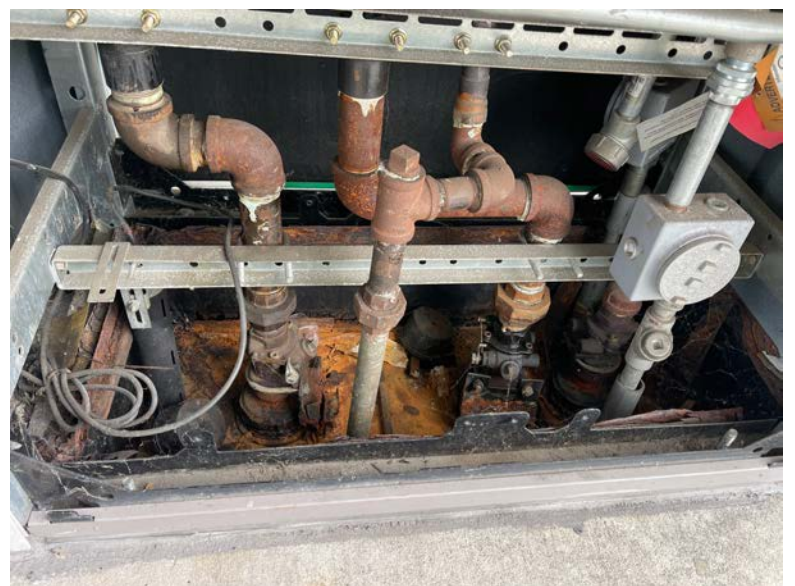
7/8 UDC and piping
