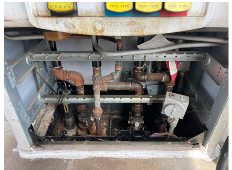
3/4 UDC and piping
