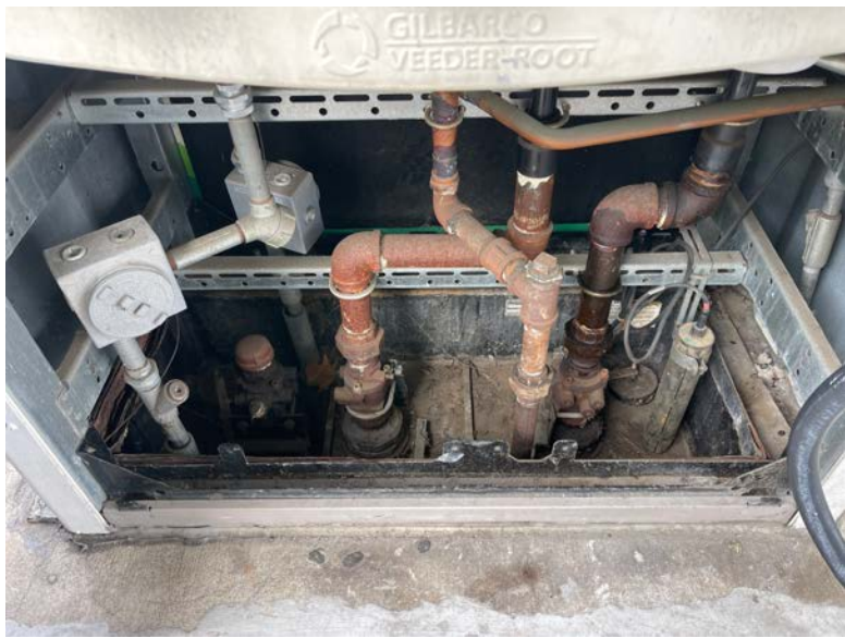
1/2 UDC and piping
